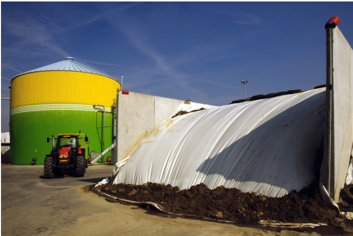
Figure 3.1: Clamp storage of feedstock at an agricultural AD facility
