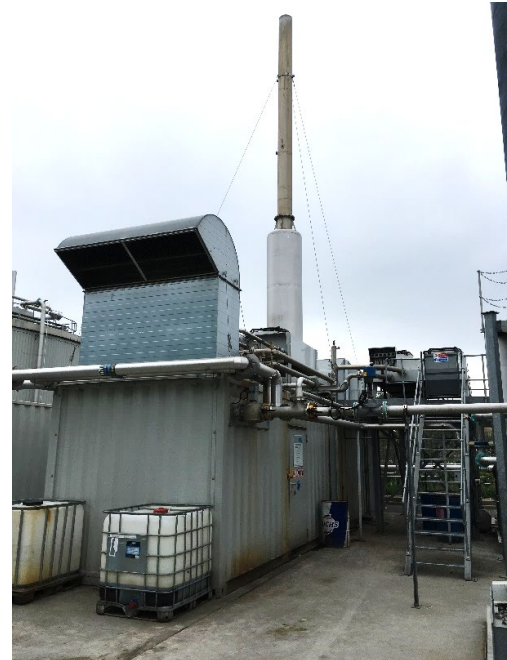
Figure 5.3: Containerised CHP internal combustion engine
